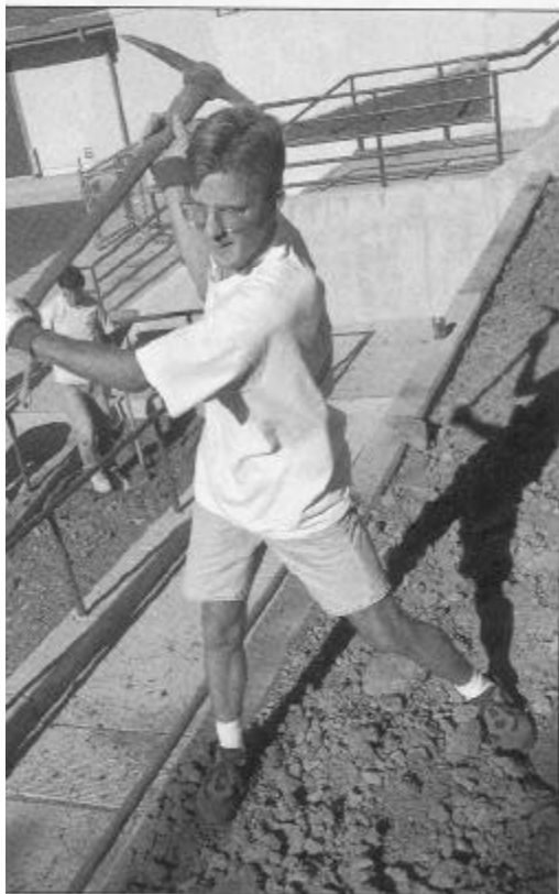
A Pacific Union College (Angwin, California) student prepares ground for landscaping at a local elementary school during a recent service day.
